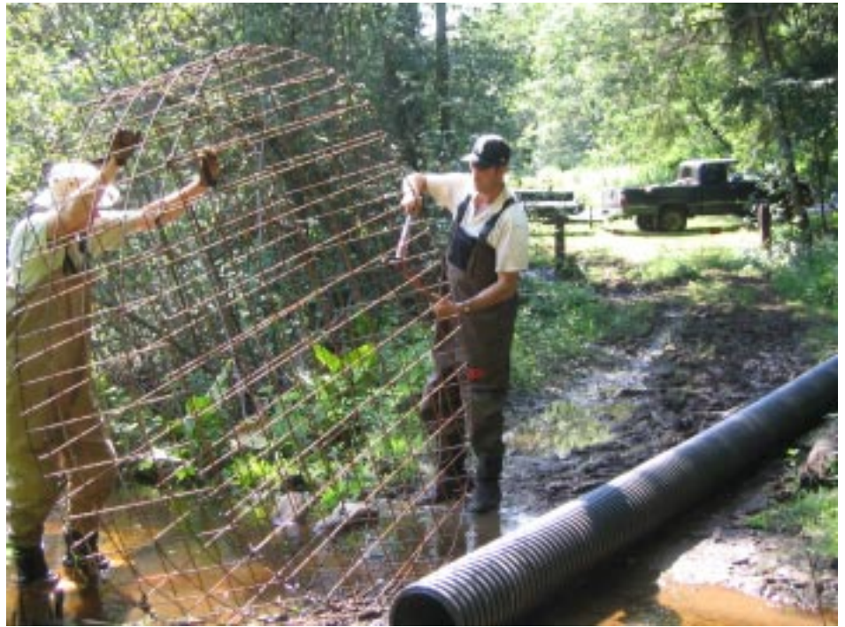
Installation of a pipe system beaver deceiver at Bradley Palmer State Park. Photo by Tracey Dejong.
