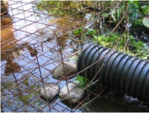
Left: Two types of flow devices known as beaver deceivers. Both were recently constructed to resolve the problem of trails flooded by beaver dams in Bradley Palmer. The top photo is a pipe flow device, the bottom uses a trapezoidal design. Photos by Tracey Dejong.
